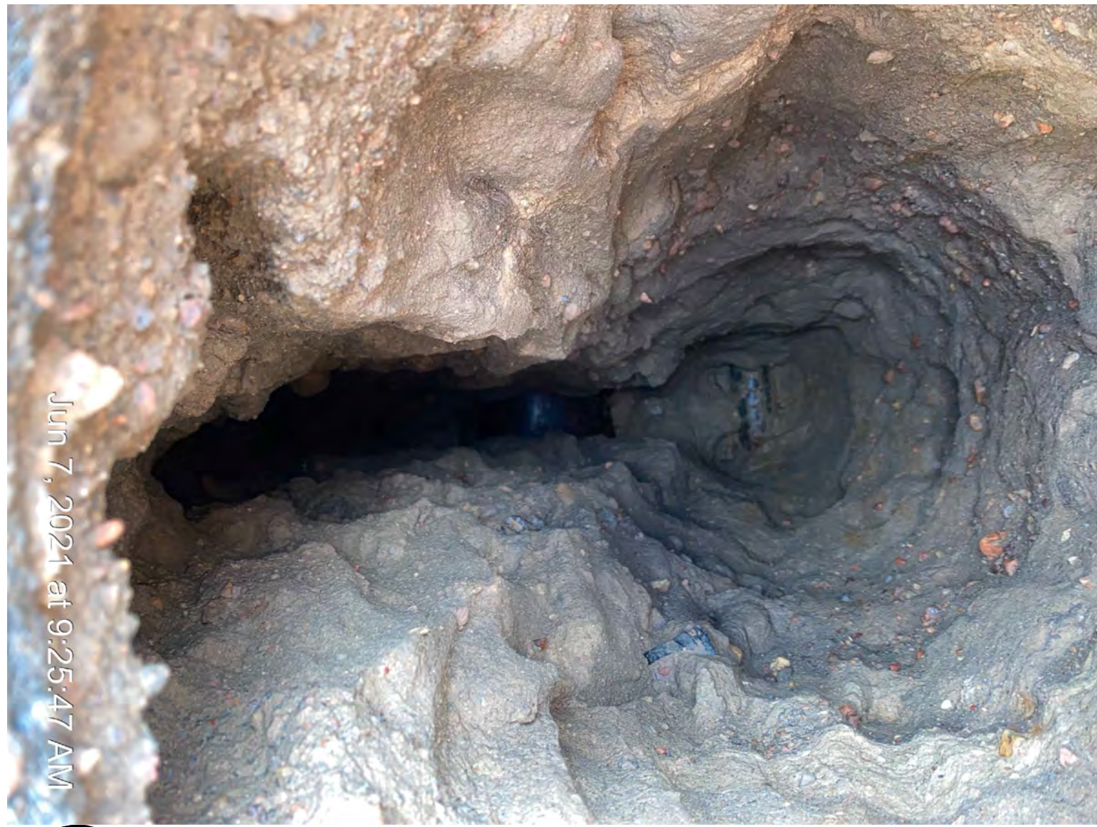
100 PHOTO OF C3D POINT #1 & #2 (POTHOLE A) SU06
